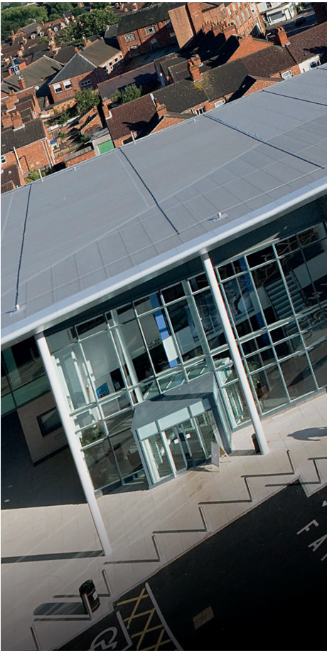
Cover image courtesy of IPS Group, North Yorkshire: Single ply membrane roof installation at the Waendel Leisure Centre, Wellingborough.
